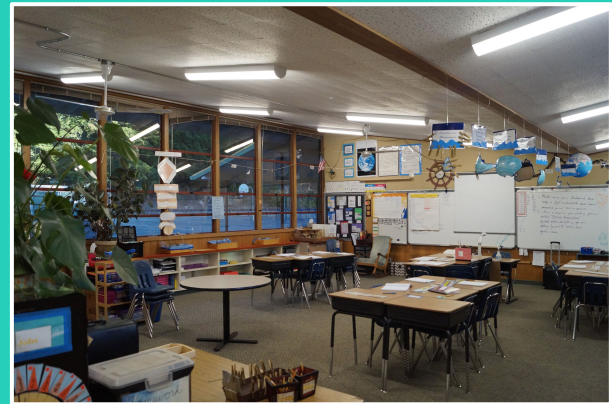
Bonny Doon Elementary LED retrofit
